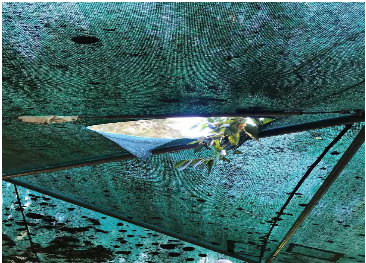
Figure 6. Displays the shade sail at with both mould and tears as a result of deterioration of the shade material.
