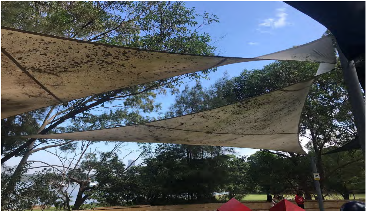
Figure 5, Shade Sails at Putney with mould build up, prior to cleaning.
