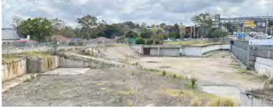
Figure 1 - Photo showing the basement of the former council building that is proposed to be filled.
