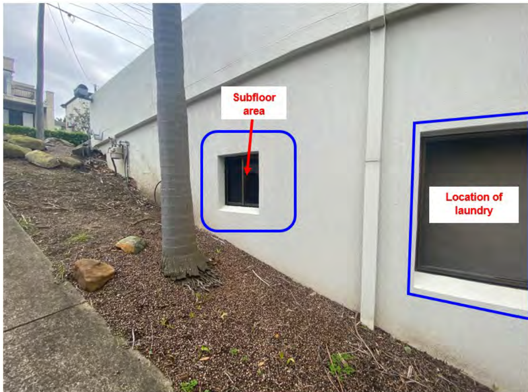
Figure 15 The location of the subfloor and laundry and bathroom at lower ground floor level as viewed from the western elevation.
